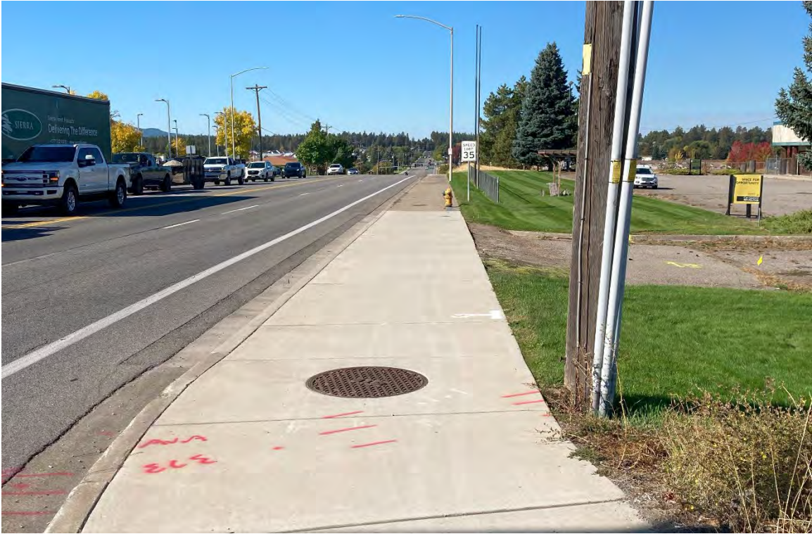
Looking west along Kathleen Avenue from the NW corner of the signaled intersection with US95: (hydrant to remain)
